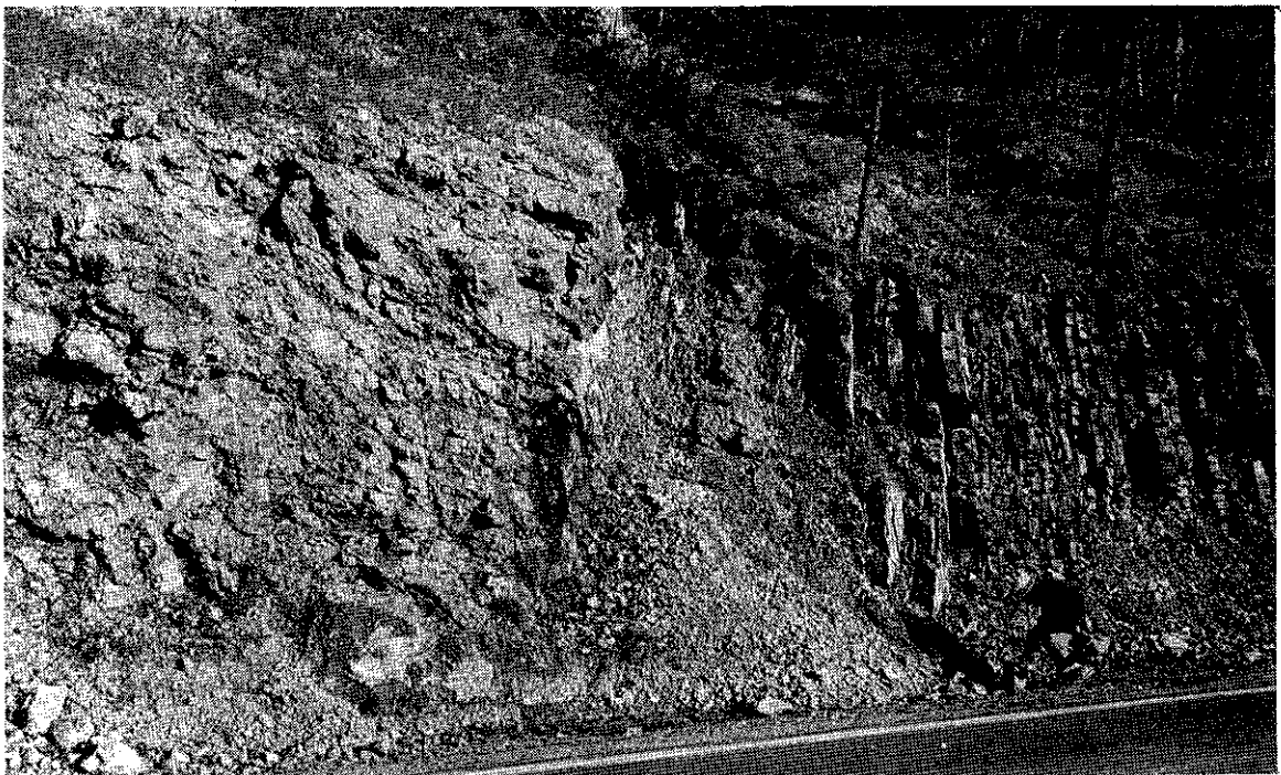
Figure 18. Stop 20. Vertical sequence of Arkansas Novaculite with altered coarse mostly novaculite breccia containing secondary manganese blebs at the top of the Lower Division (to the left), overlain by thin, often graded, chert and shale with some turquoise coatings in the Middle Division near the north central part of the Caddo Gap section on Arkansas Hwy. 27.
